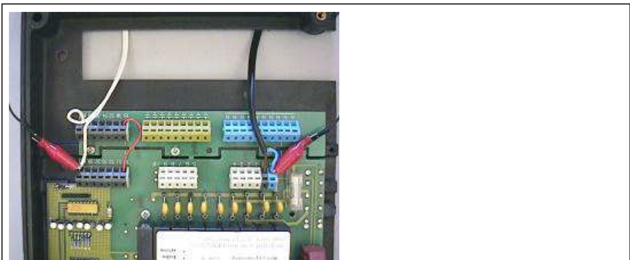
Figure 24: Injection of disturbance current into the device under test via a two-pole connection and a galvanic isolating point.
